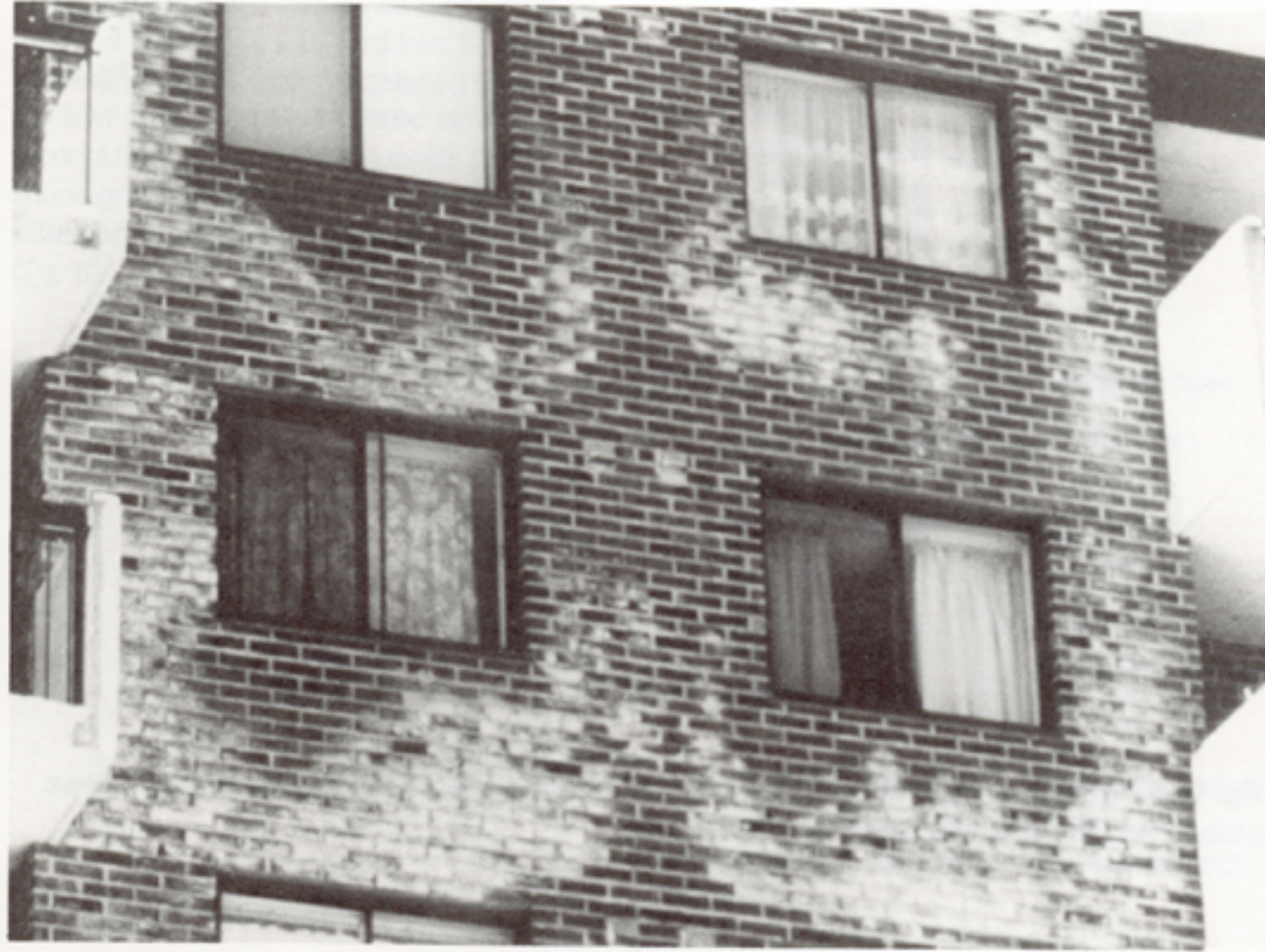
Fig. 16 An example of extensive wetness and efflorescence
