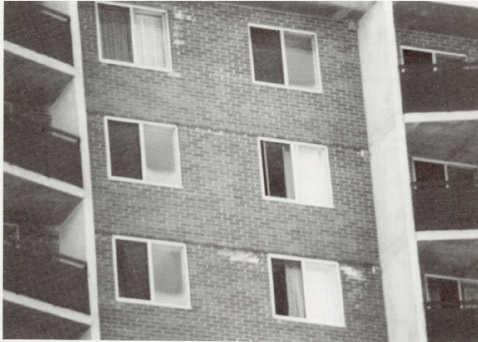
Fig. 15 Example of air leakage on the side of a building
