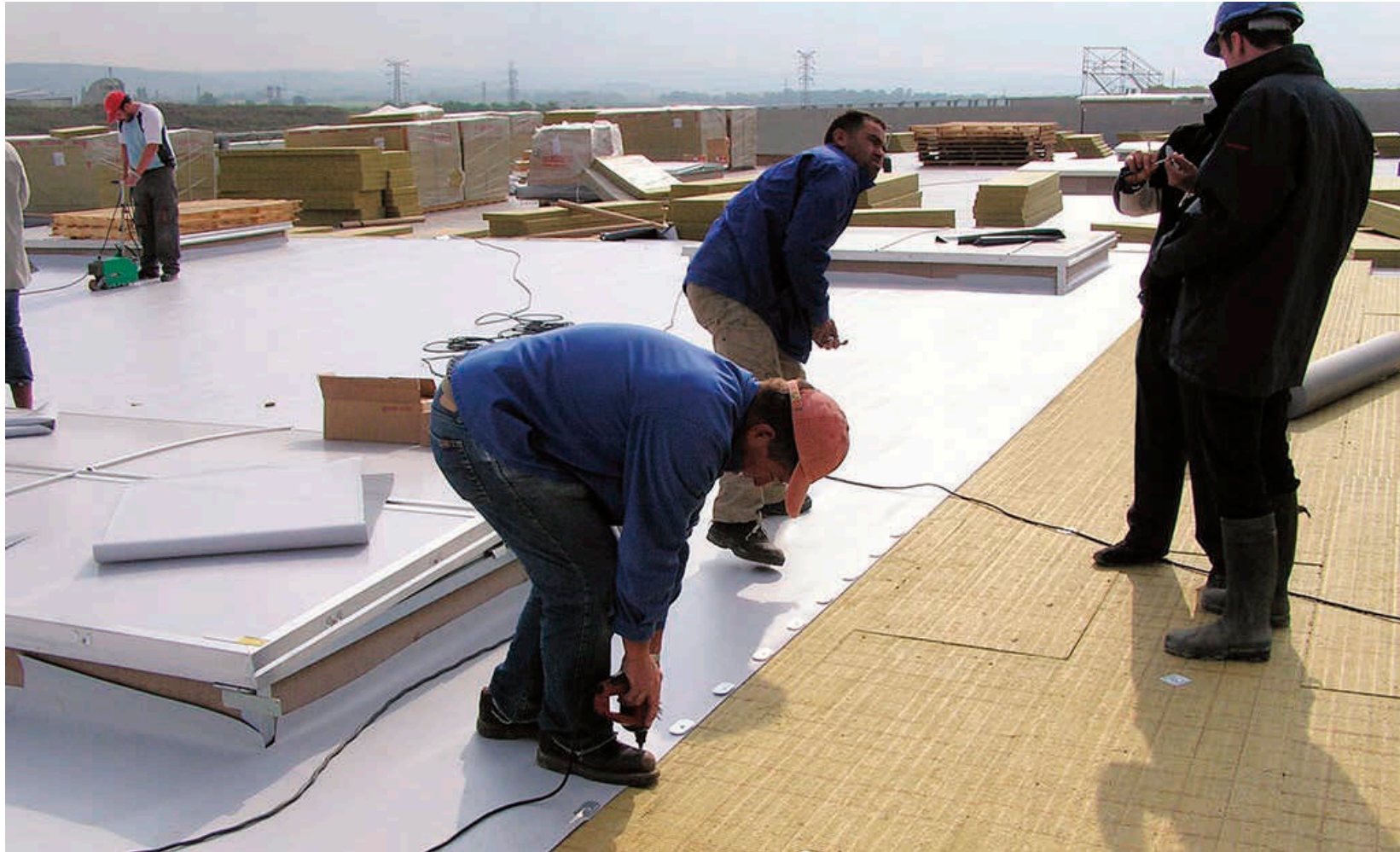
Roofing membrane is being installed over the dense/rigid rockwool insulation to protect it from moisture.
