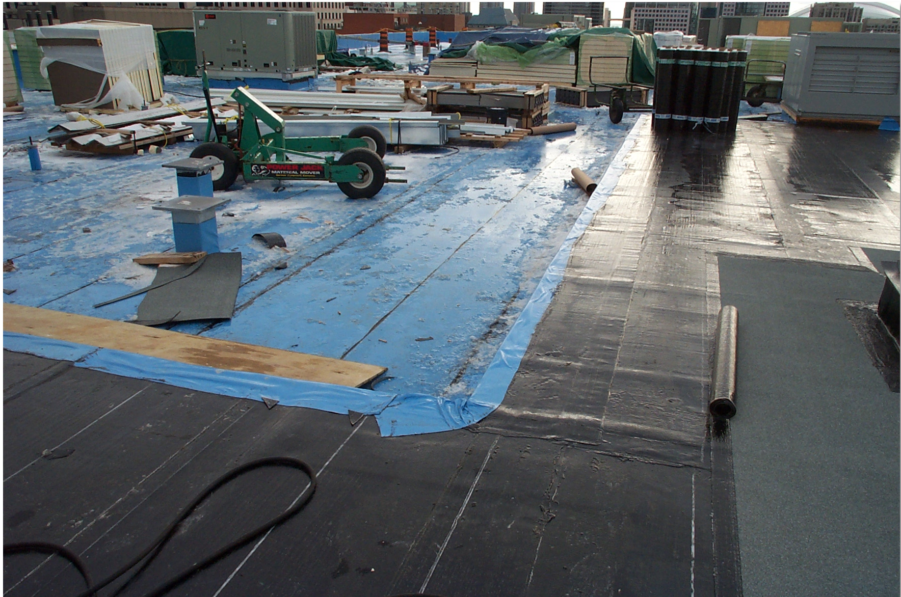
This is a multi-ply installation. The black being the base layer and the grey the more durable top layer. The insulation is beneath the black layer.
