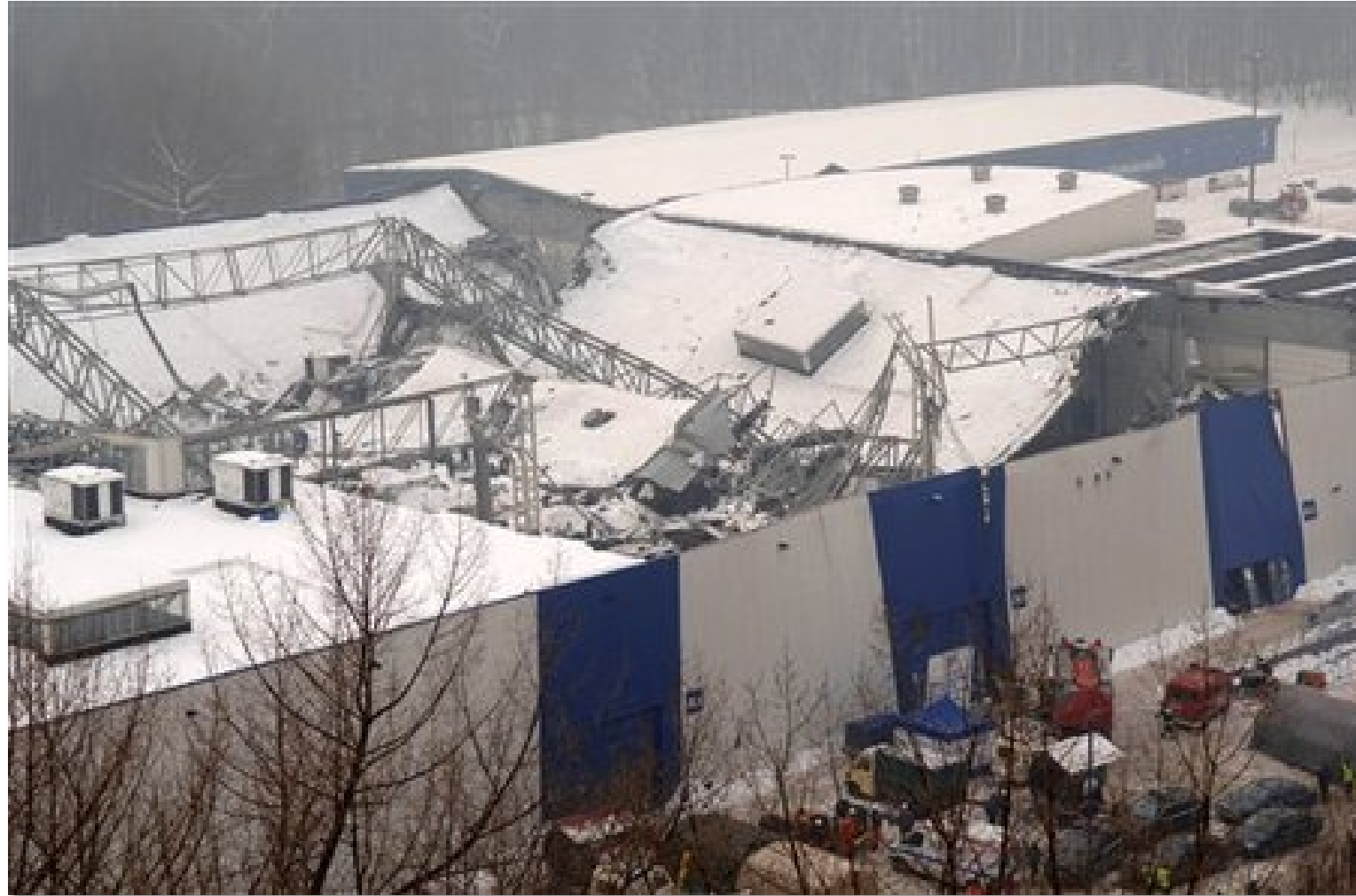
Roof collapse in Poland due to excessive snow loading
