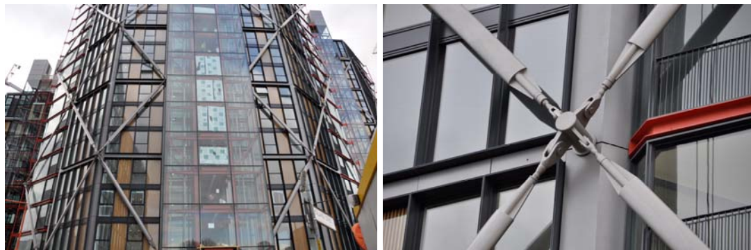
Figure 12: An external bracing system is used on the NEO Bankside housing project in London, England by Rogers Stirk Harbour and Partners. Although not designed for seismic resistance, the bracing system is proudly exposed and a critical part of the aesthetic of the building.
