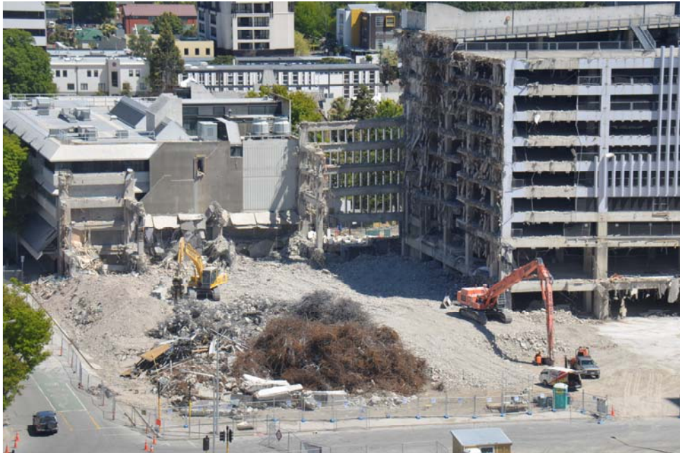
Figure 1: View of Christchurch Central Business District, November 2012. The demolished reinforced concrete has its rebar separated for recycling.
