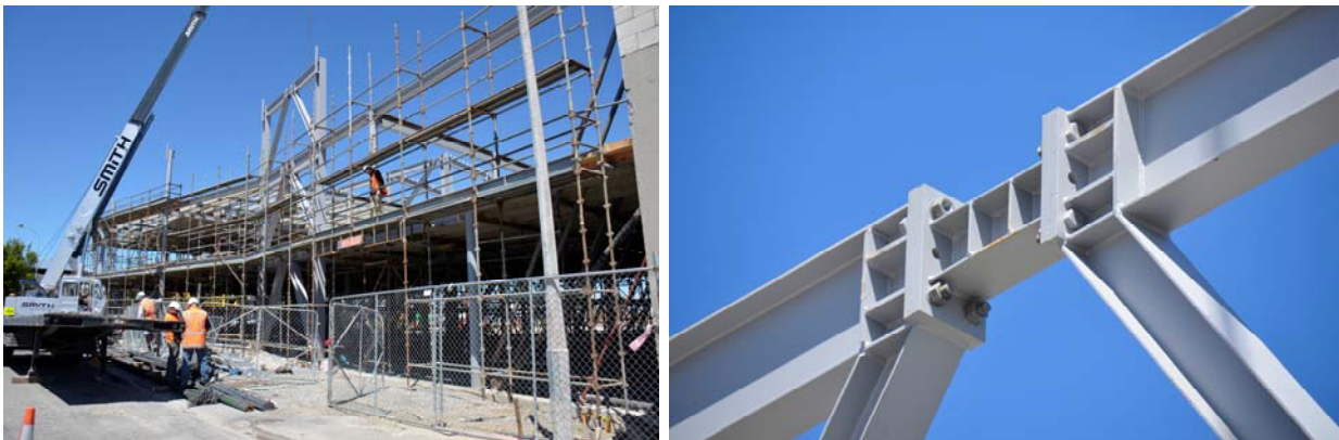
Figure 7: A braced frame in the Three35 Project that uses a "replaceable link" in post earthquake construction in Christchurch.
