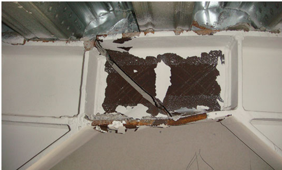
Figure 2: Fracture in an Eccentrically Braced Frame in the Pacific Tower. Courtesy of Sean Gardiner, CPG New Zealand Ltd.
