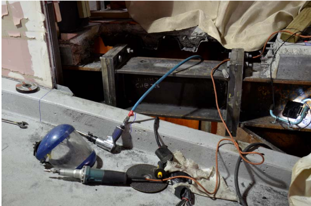
Figure 3: A link element in a braced frame in Pacific Tower. Note that the wall had to be torn away to provide access to the joint, and the access is still not ideal for labour.
