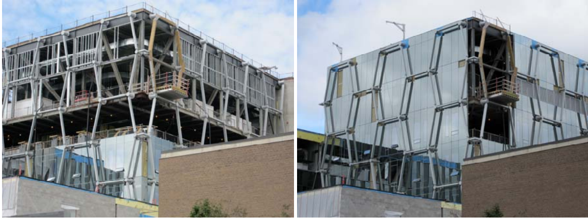
Figure 11: A system of exterior bracing is used on this laboratory building at the University of Waterloo in Canada, designed by KPMB Architects.
