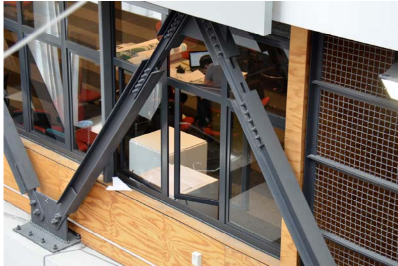
Figure 9: This retrofit bracing is located in the atrium of the School of Architecture in Wellington, New Zealand. These innovative braces are using fairly standard, tested, section types but creating a different sort of bolted link section. They have become a key aspect of the architectural aesthetic of the space.
