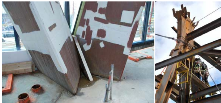
Fig. 5: The nodes on the Bow Encana are of two types. The diagrid on the south façade (left) is expressed as part of the double façade atrium and has been designed to AESS4 standards. 7 The node-to-diagonal connections were welded. The diagrid on the north façade (right) is concealed so although the connections have also been welded, the system is constructed of different section types and to a Standard Structural Steel level of finish.
