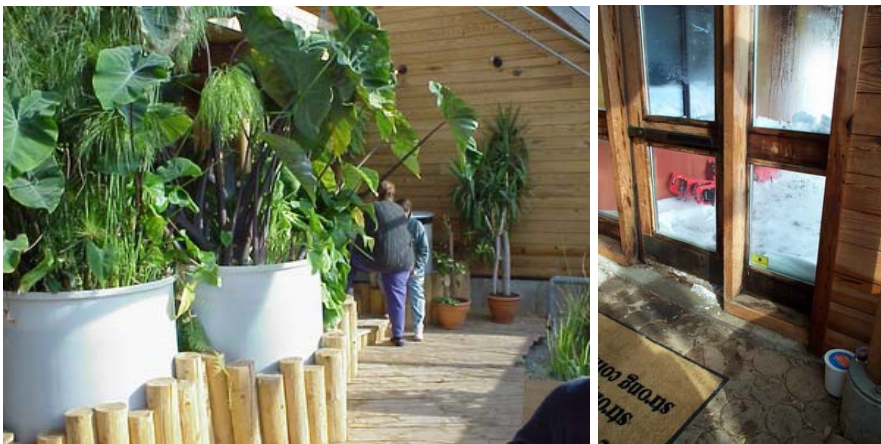
Figure 3: YMCA Environmental Learning Centre, Charles Simon Architect Water Efficiency: Credit 2 Innovative Wastewater Technologies: Living Machine™ – adjacent doors suffering from deterioration due to the high moisture content of the room
