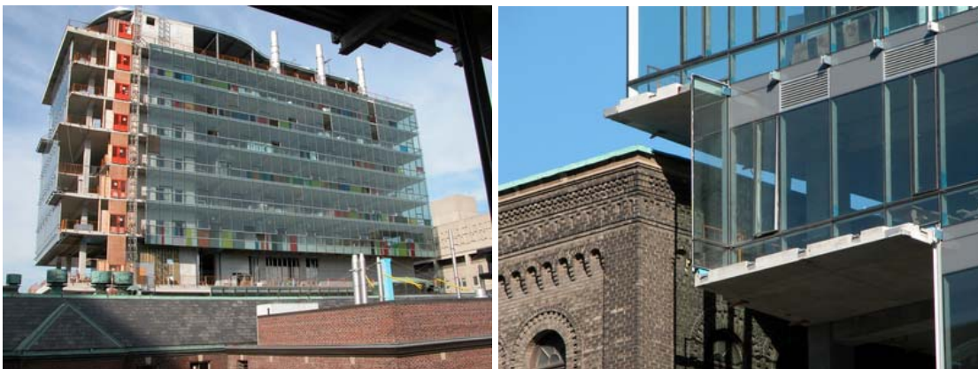
Figure 11: Innovation and Design Process: Centre for Cellular and Biomolecular Research, University of Toronto, Benisch and Benisch. Double skin façade construction in progress. The building also uses innovative planning to separate less climate controlled corridor spaces from highly controlled laboratories. Two storey planted atriums will be located at the corners of the south face of the building.
