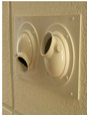
Credit 2: Increase Ventilation Effectiveness - directional air vents aid displacement ventilation
