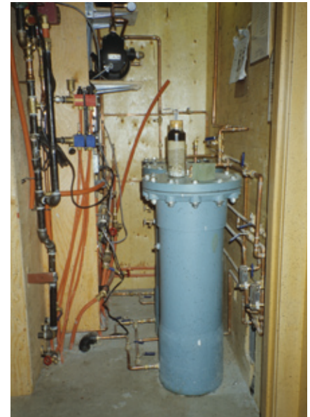
◀ CMHC Healthy House Close up view of PV screen suspended from balcony railing, ▼ Healthy House Waterloo Biofilter unit in a closet. Photo: http://www.architecture.uwaterloo.ca/faculty_projects/terri/cmhc.html
