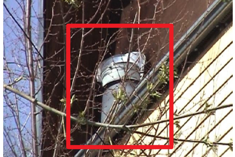
Figure 22: “Light scoops” help bring natural light deep into the house, on all floors.
