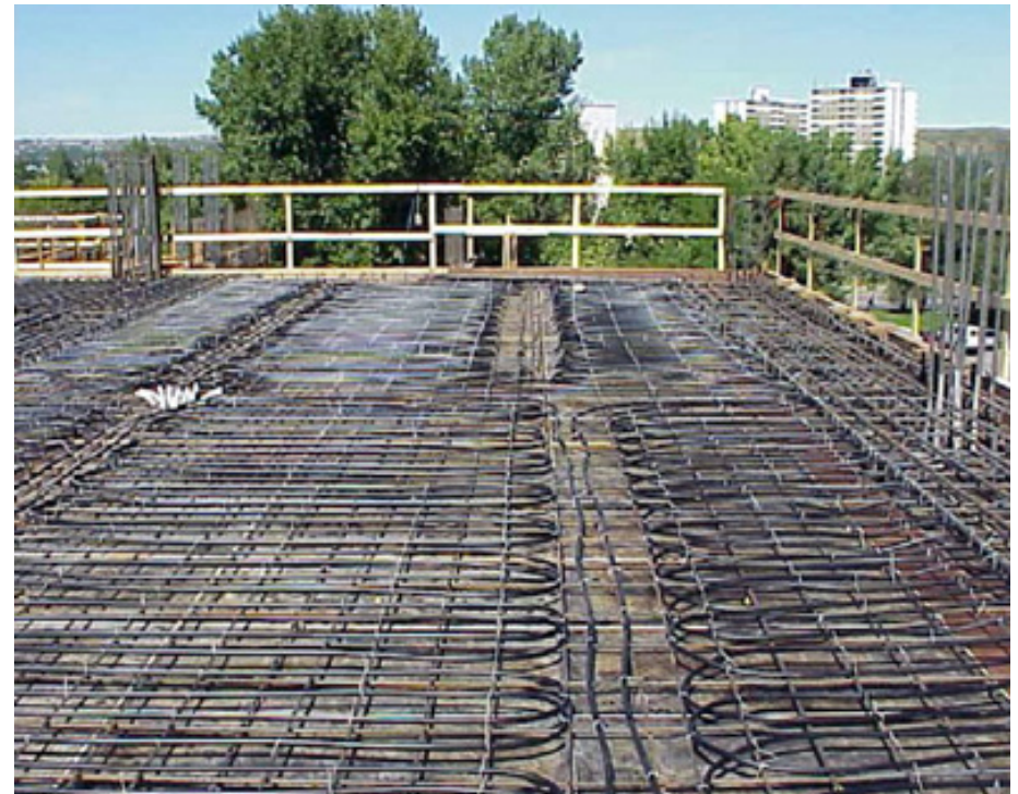
Below: Hydronic pipes are carefully laid, and secured to rebar prior to the pouring of the concrete slab.
