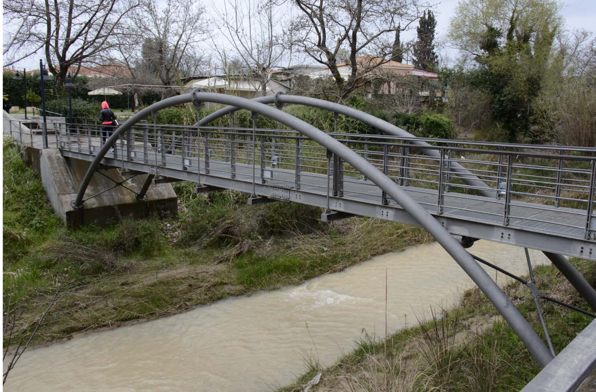
Bridge coated with a zinc rich paint which is holding up well but the bolts are inferior and are rusting.
