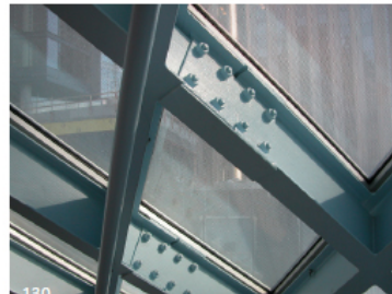
130 This building uses extensive diagrids formed with I sections. These are very simply attached using bolted splice plates on both sides of the flange.
