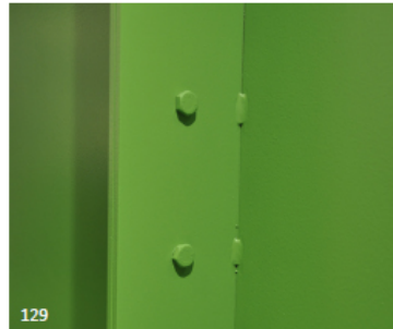
129 This connection has taken care to align the required intermittent welds with the bolts. This avoided unnecessary welding or filling.
